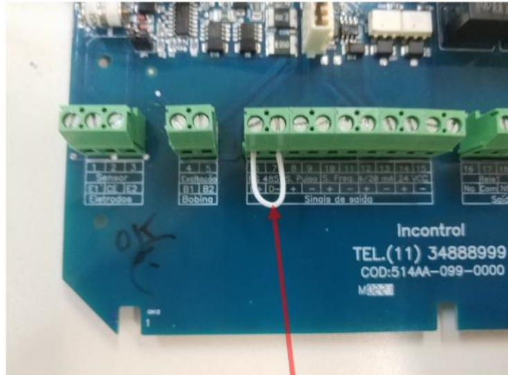
Jumper instalado na Porta RS485
